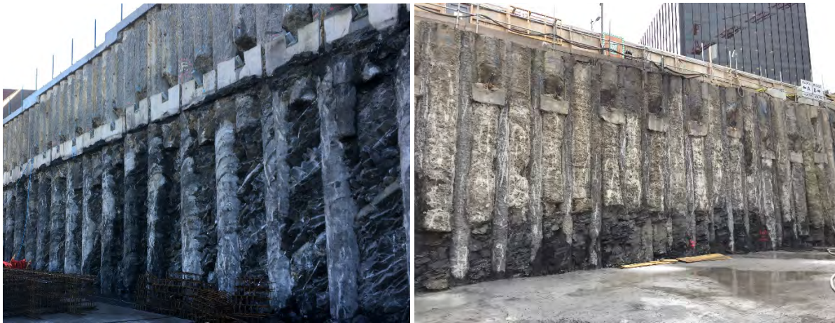
Figure 4 – Typical secant arrangement within rock formation (Murphy International Ltd. & PJ Edwards & Co. Ltd.)
